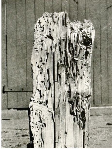
Douglas fir pile destroyed by marine borers. Hill and Kofoed, Marine Borers and Their Relation to Marine Construction on the Pacific Coast , 87.
